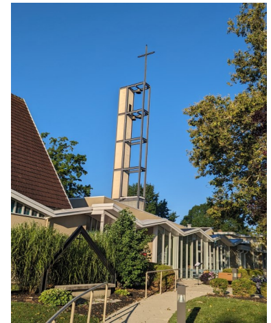
The bell tower is in need of extensive repairs.
